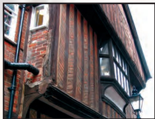
Detail of the brickwork in the remaining part of Jack's house in Northbrook Street.
